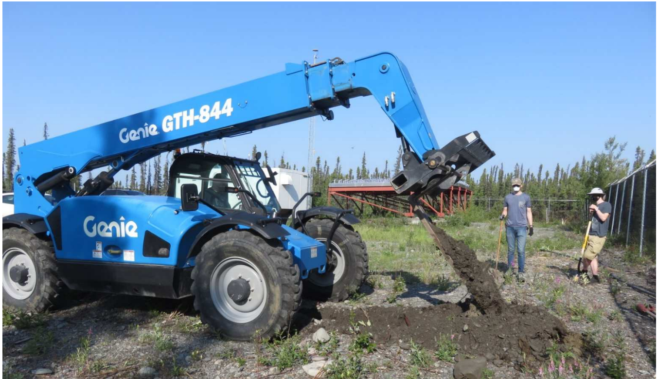
Figure 16 ~ The ground was too rocky for a power auger, so a fully articulating forklift was used to open a short trench for the sensors. The forks were rotated to a vertical position, rammed into the ground and then rotated to scoop out the soil. No water was encountered to a depth of about 1.5 m (5 ft) but wood residue from the original site clearing was found.
