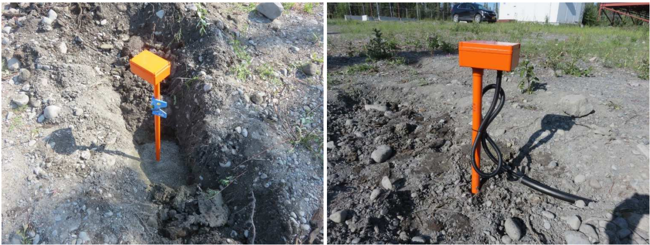
Figure 18 ~ The area around the sensors in the trench was backfilled with a layer of pea gravel followed by six 60 lb bags of traction sand. After backfilling, the connectorized cable was connected to the sensor junction box and the system placed into service.
